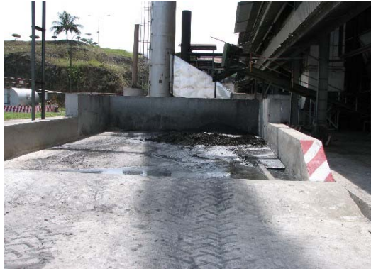
Plate 2: Boiler Ash Containment Bund
